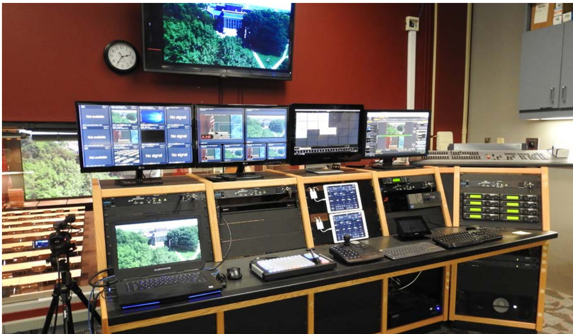
New Control Center above Sellers Auditorium
